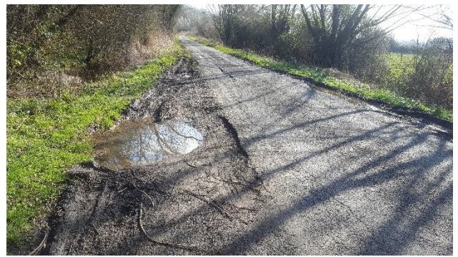
Informal passing place with signification deterioration
